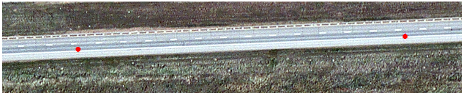
Mile 114.3-114.4, Fatigue 6578 square meters
