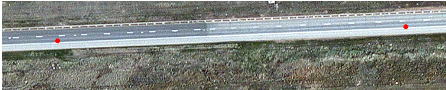
Mile 114.2-114.3, Fatigue 3250 square meters
