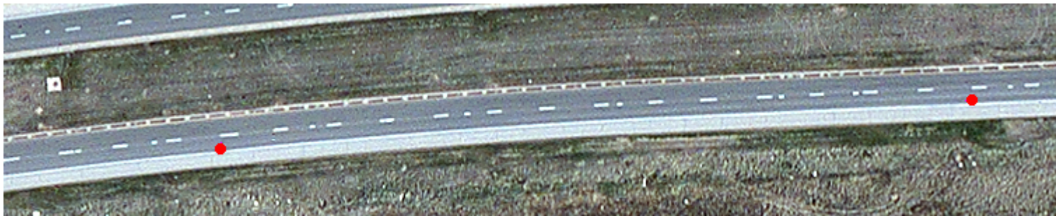
Mile 114.1-114.2, Fatigue 414 square meters
