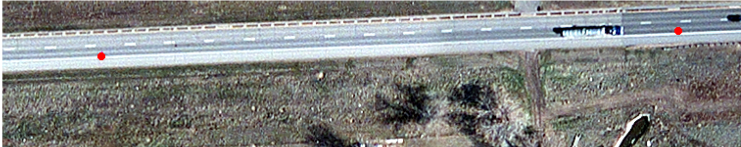
Mile 114.4-114.5, Fatigue 6578 square meters
