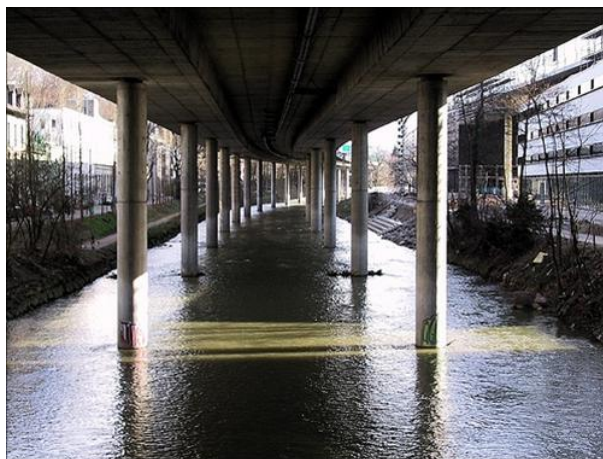
Figure 7. The Sihllochstrasse bridge selected as bed site for its size and its structural complexity.
