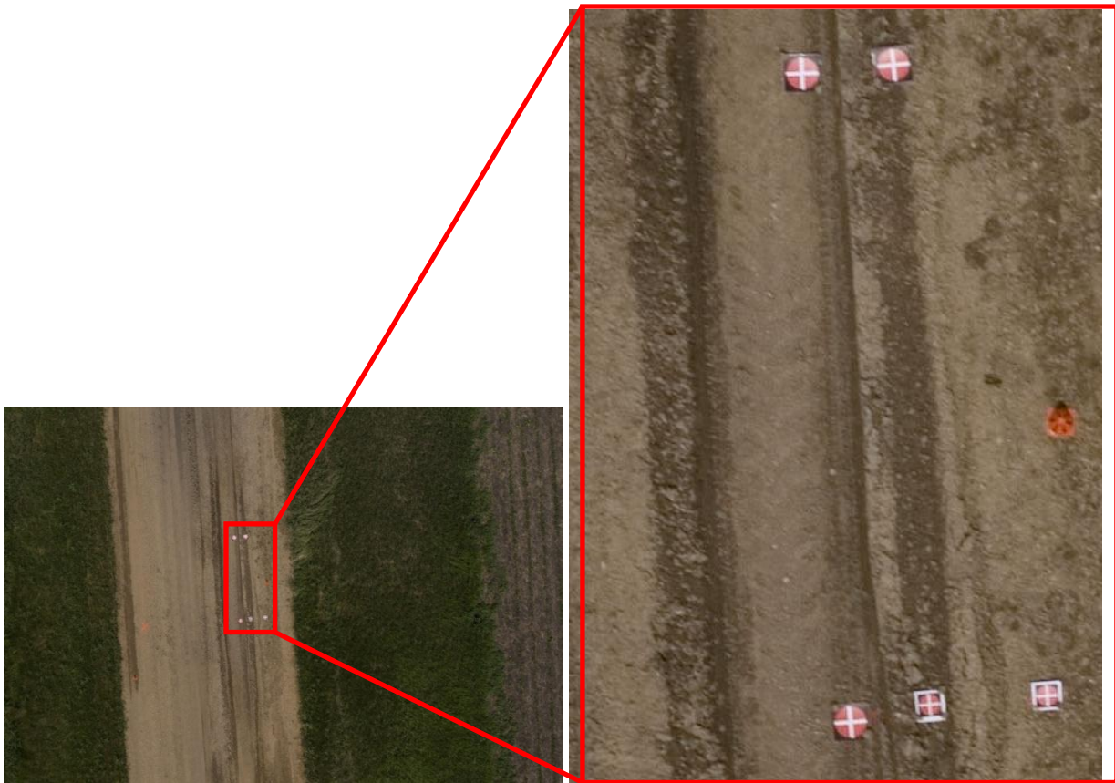
Figure 19. Road image acquired by UAV showing severe ruts. Note the marks are designed for ground measurements and for relating ground measurements with image measurements.
