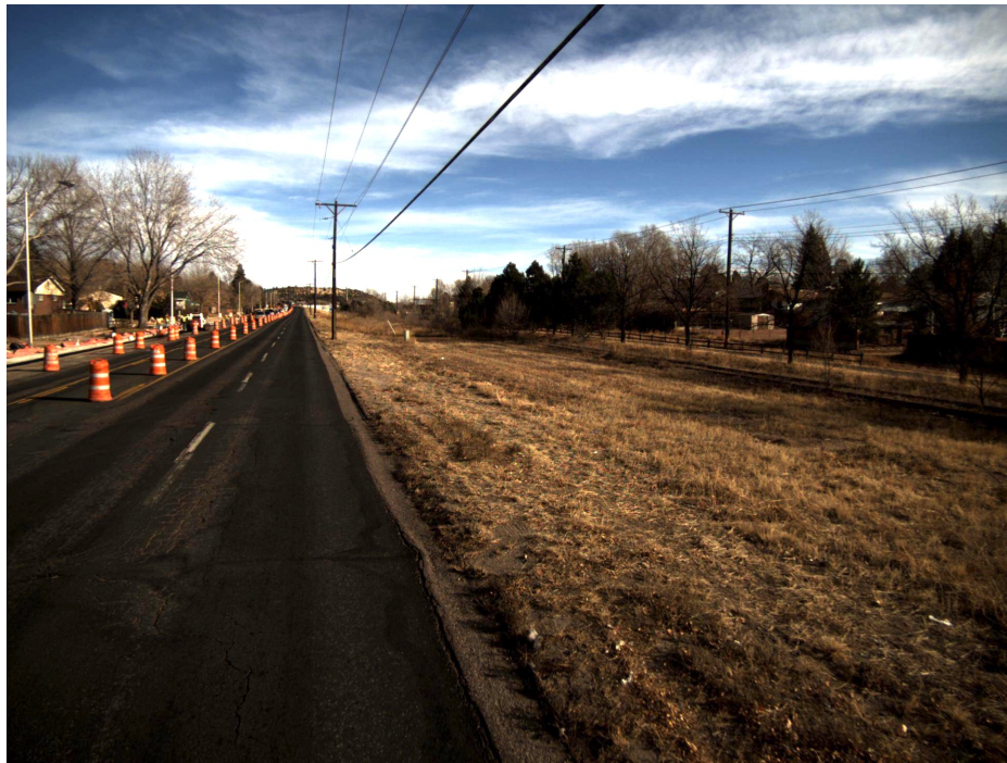
Figure 16. A photograph of Constitution Ave. and Wynkoop Dr. in Colorado Springs. Obvious road fatiguing can be recognized.
