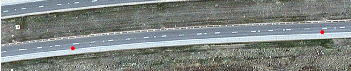
Figure 5. Aerial imagery Mile 114.1-114.2, Fatigue 414 ft 2
