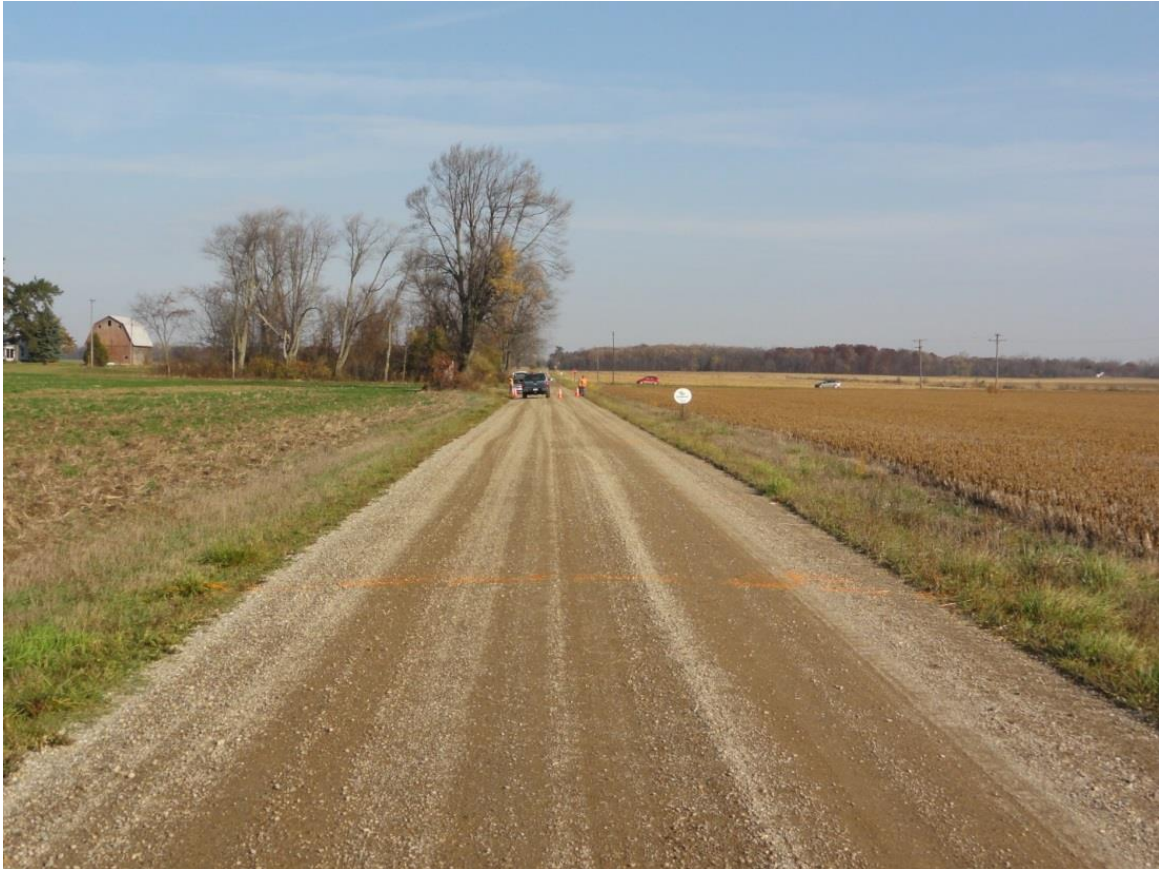
Figure 18: Mills-Macon Road south of Welch Road looking north. Note thin layer of loose aggregate on the road surface and lack of other distresses on the road surface. (DSC03667)
