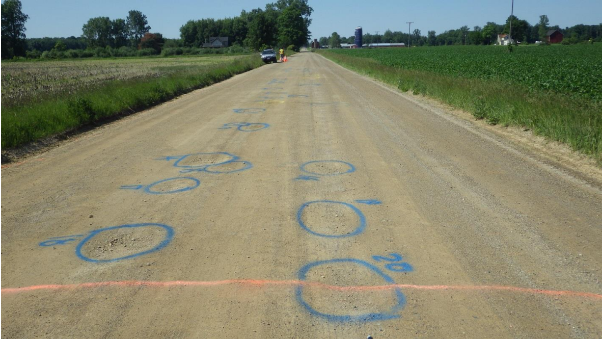
Figure 32: Distress markings on analysis segment 2, Fleming Road, Livingston County MI. Each distress feature was circled and numbered when it was mapped.
