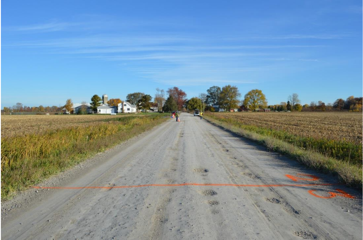
Figure 12: Petersburg Road near Milan MI looking north. Note visible distresses (potholes).
