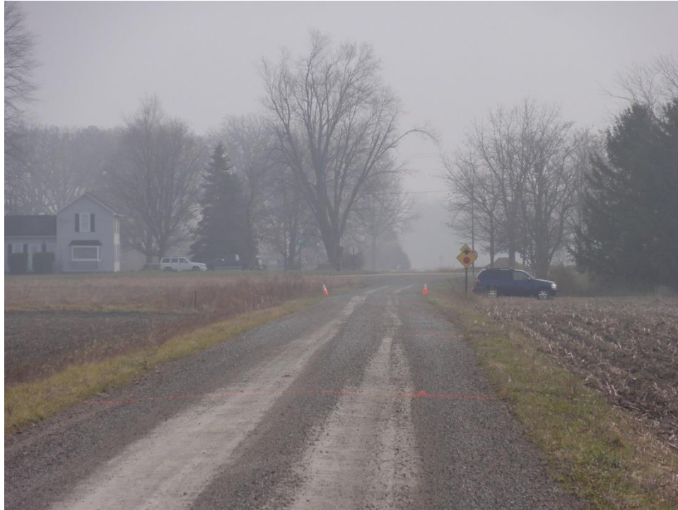
Figure 26: Garno Road looking east. Note the loose/float aggregate on the road shoulders and along the crown of the road.
