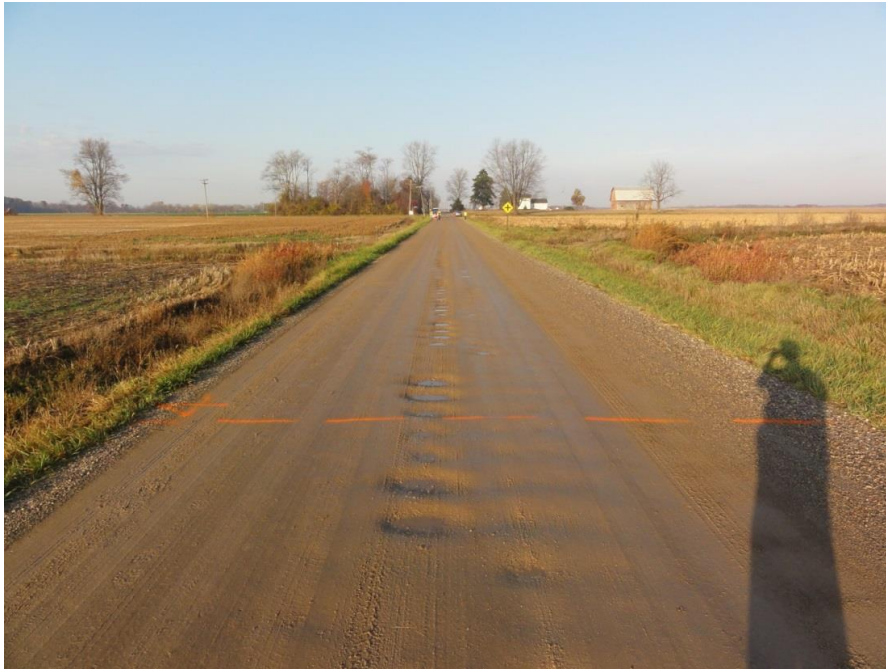
Figure 14: Welch Road (facing west) near Mills-Macon Road, Lenawee County, MI. Road segmentation marks, potholes, washboarding (corrugation) and float aggregate are visible in this image. (DSC03546)
