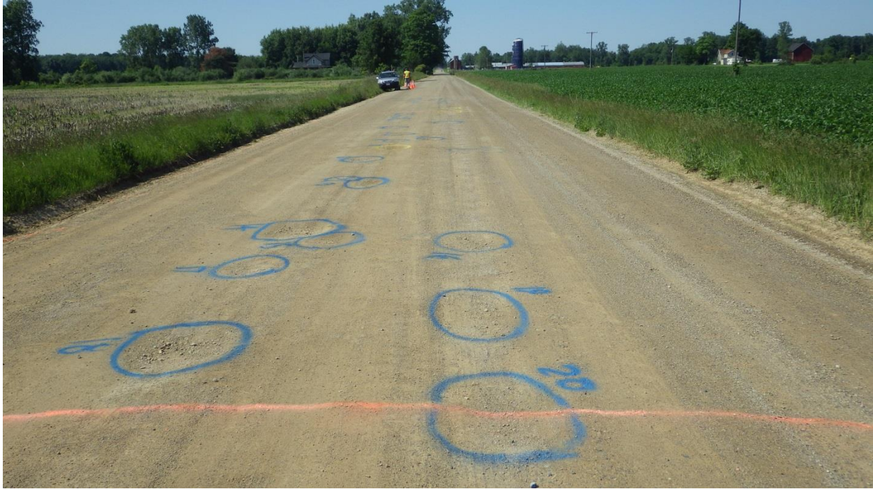
Figure 8: Fleming Road segment 2 looking north. Distresses have been marked, measured, mapped and numbered prior to overflight. This image correlates to the south end of the distress map above.
