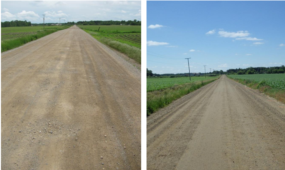
Figure 30: Marsh Road, north of Fowlerville, Livingston County, MI looking south. Image on the left illustrates some of the distresses present on May 31, 2013; the image on the right was taken June 18, 2013. (IMG_4890 (L); IMG0030 (R))
