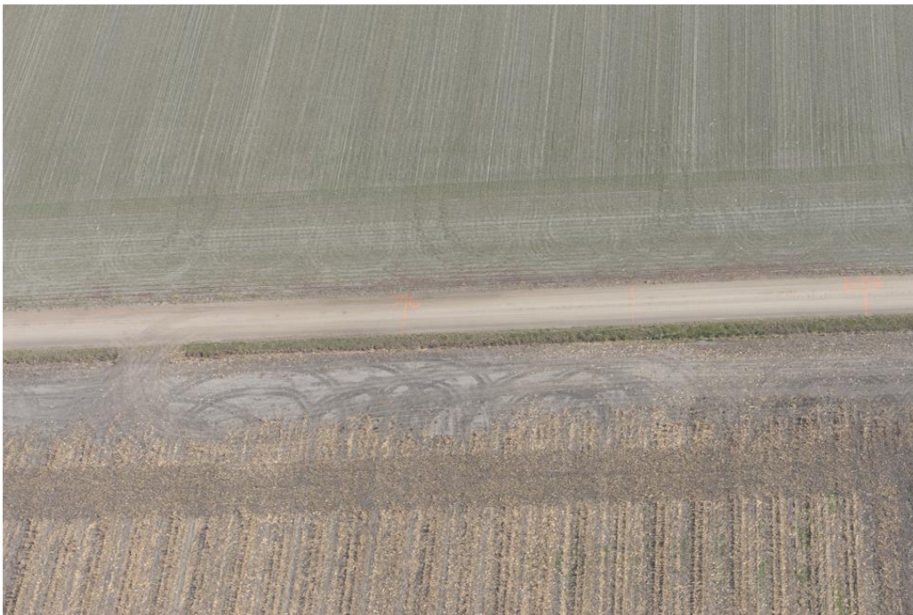
Figure 23: An aerial view of segment 6 of Piotter Rd from a Cessna 172 flying at approximately 500 feet above ground level. The orange segment marks are clearly visible, but distresses are difficult to identify from this angle and altitude. (DSC5879)
