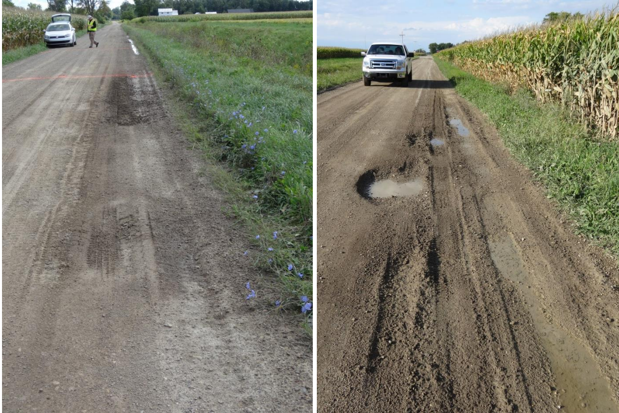
Figure 39: Ruts and potholes on Palmer Road. Note deformation along edge of road in left hand image. DSC00691 (R) and DSC00717 (L)
