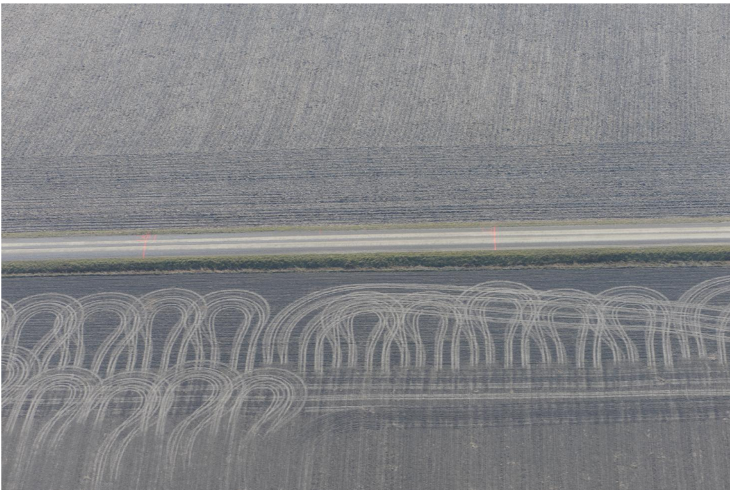
Figure 28: Garno Road from a manned fixed wing aircraft at approximately 150 m / 500 feet agl (above ground level). The float aggregate distress is visible, but not easily characterized from this angle and altitude.
