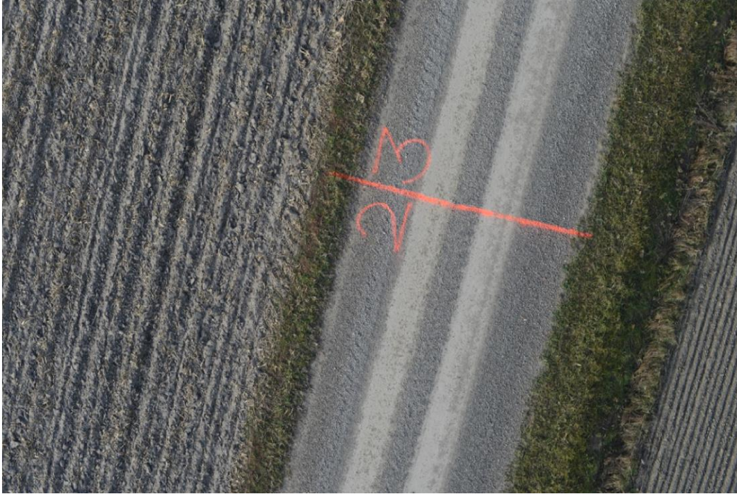
Figure 27: Garno Road from the MTRI helicopter at 25 meters. Loose/float aggregate is the only distress present. Note the marks in the loose gravel from the tires of farm equipment.
