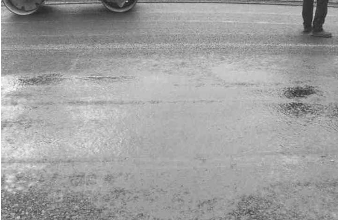
Figure 4.1 Bleeding of Bottom Ash Pavement.
