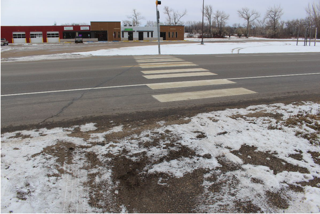
Figure 5.3 Missing ramp near Four Winds High School
