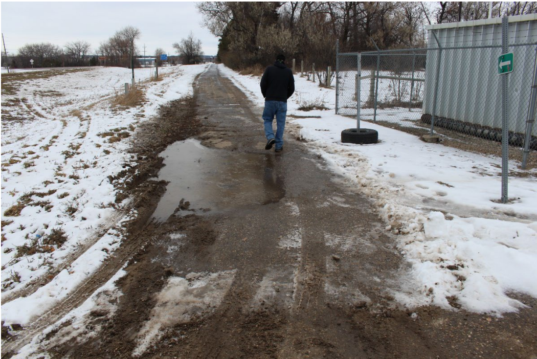
Figure 5.8 Puddle of water on damaged sidewalk
