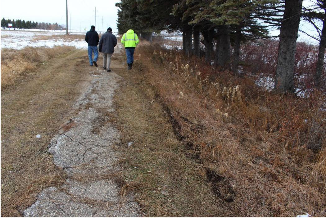
Figure 5.9 Weathered sidewalk and weeds
