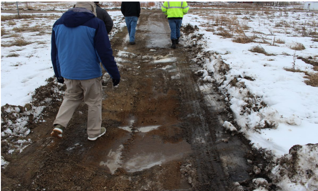
Figure 5.2 Discontinuity in sidewalk
