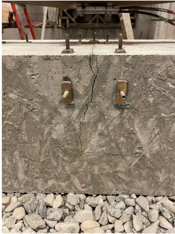
Figure 5.10 Control Slab Initial Crack
