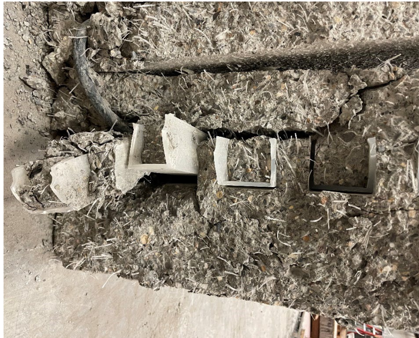
Figure 5.22 FRC Slab Exposed Failure Plane
