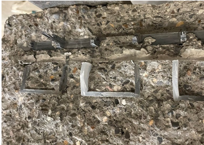
Figure 5.24 FRP Grid Slab Exposed Failure Plane
