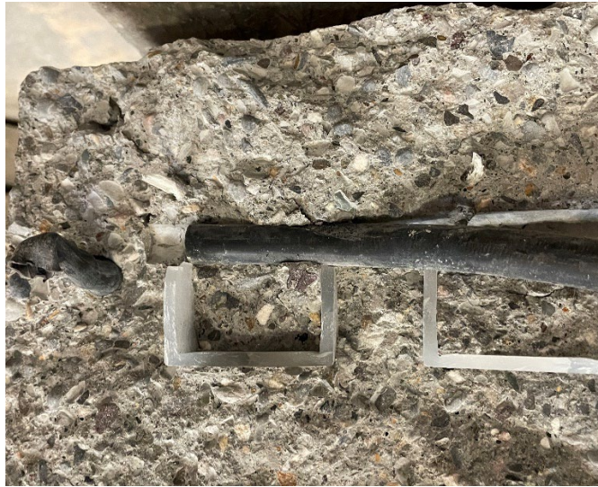
Figure 5.23 GFRP Rebar Slab Exposed Failure Plane
