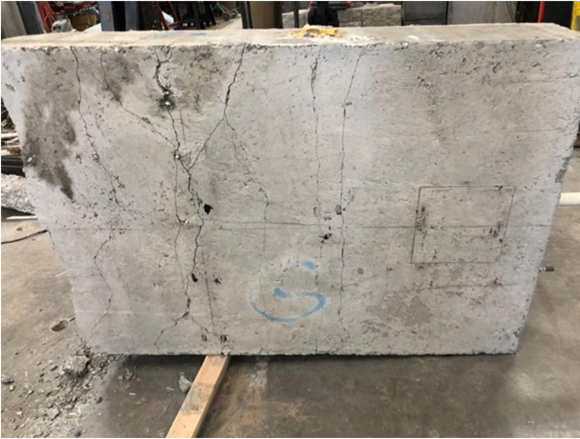
Figure 5.23 Face of GFRP Reinforced Slab After Failure
