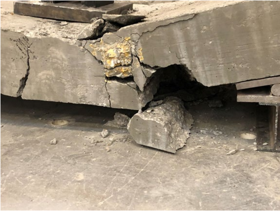
Figure 5.9 Spalling Slab with Steel Reinforcement
