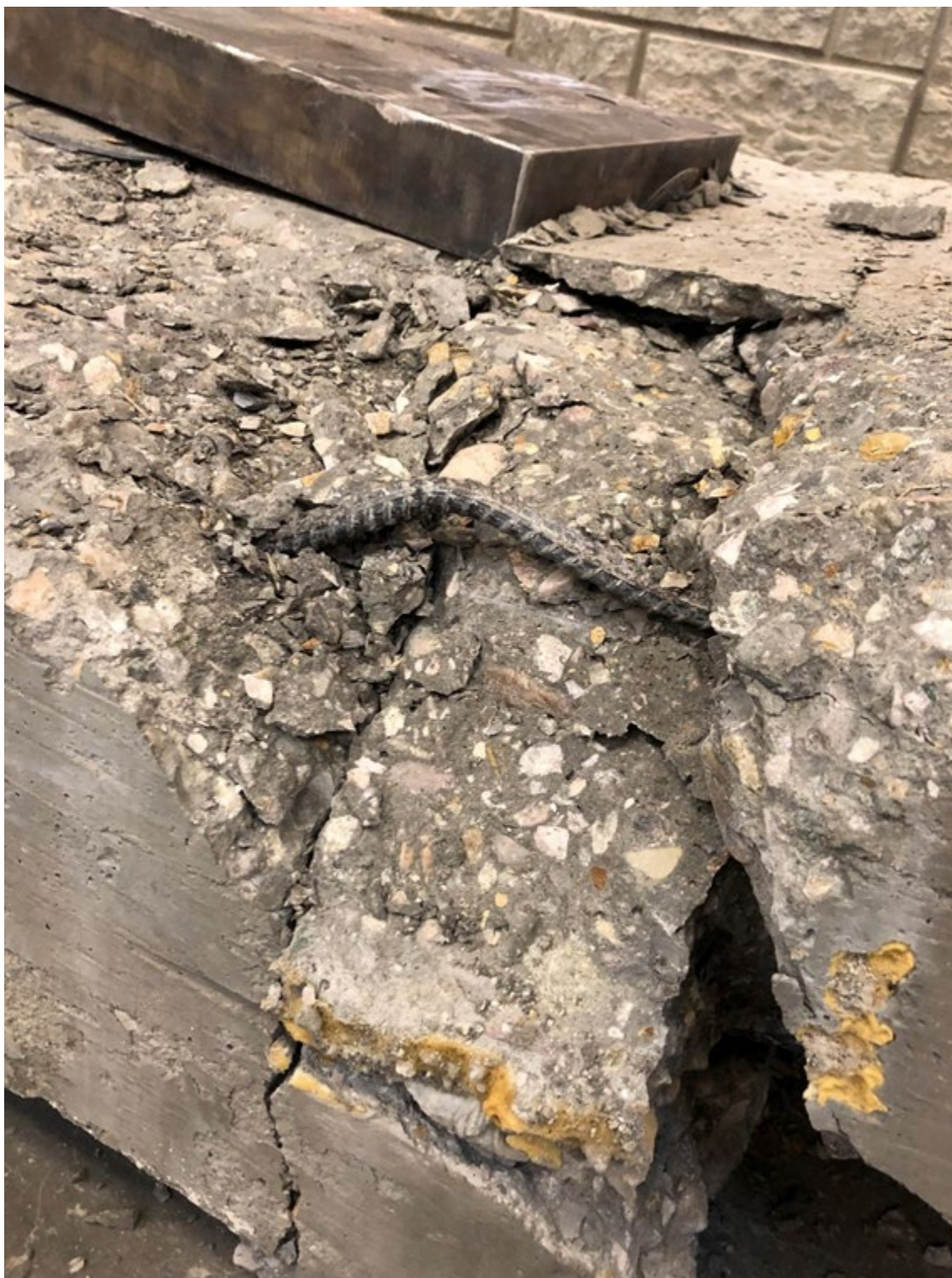
Figure 5.11 Steel Reinforcement Failure
