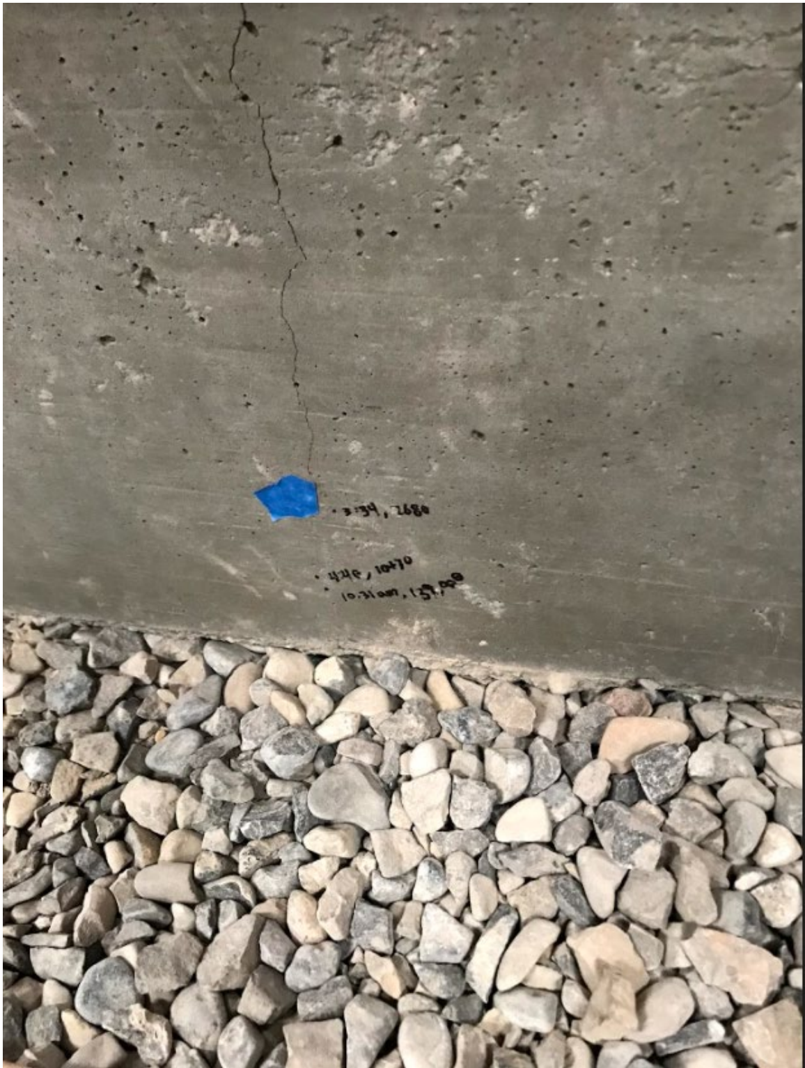
Figure 5.16 GFRP Side Cracking
