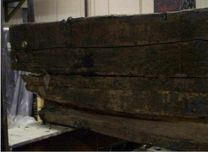
Figure 5.15 Splits and checking visible on side of Specimen 3
