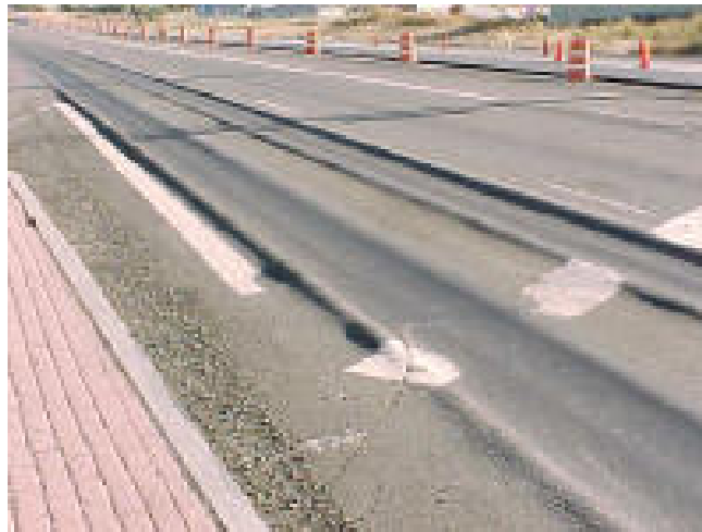
Figure 2.3 Rutting in Pavement
