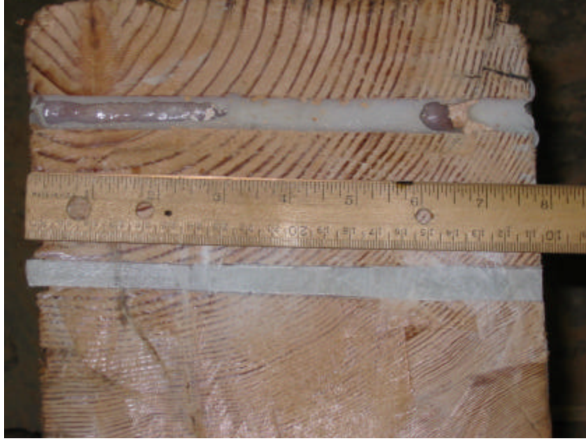
Constant 12.7mm (0.5 in.) diameter hole throughout the depth of the beam with no shear spike present.
