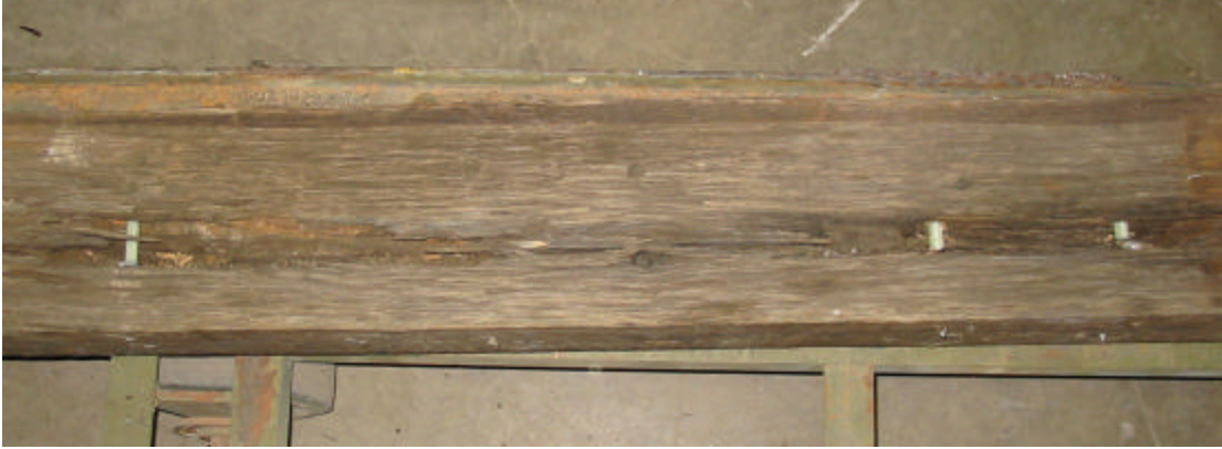
Figure 12. Large decay voids reinforced with shear spikes
