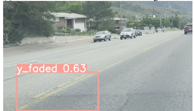
(h) Faded Yellow Double Lane Marking
