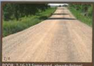
7/4 POOR: 7-16-13 Same road, already failing!
