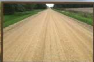
GOOD: Residential road, initial treatment 0.5 gal per sq yd. Same treatment year 2. Gets 0.25 - 0.3 gal treatments in succeeding years. Treated annually 10 yrs. Performs very well.
