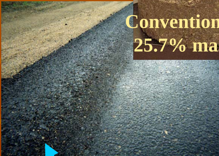
Raveling in the field
